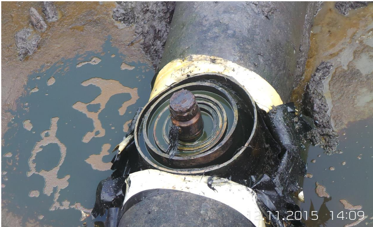
Fig B: Valve was cut and coned
