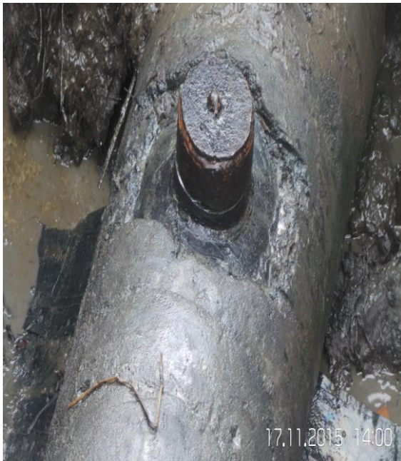
Fig B: Spill point after excavation
