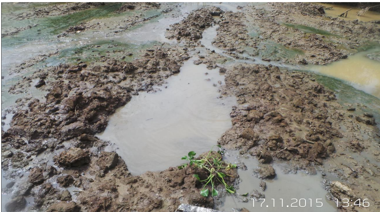
Fig A: Spill point just before excavation
