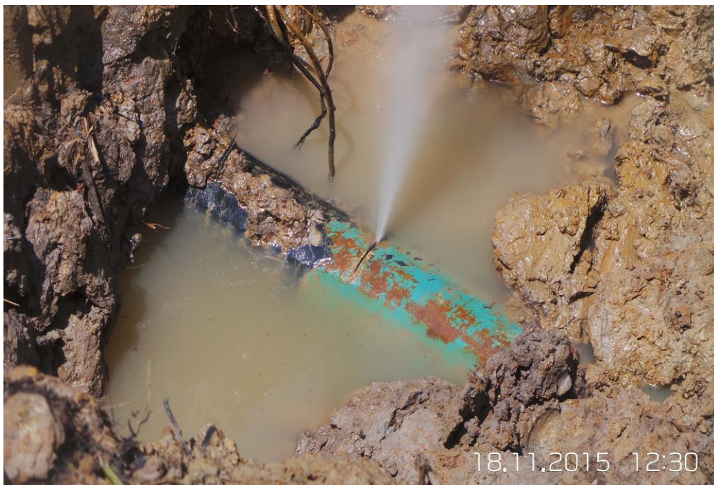
Spill point after excavation
