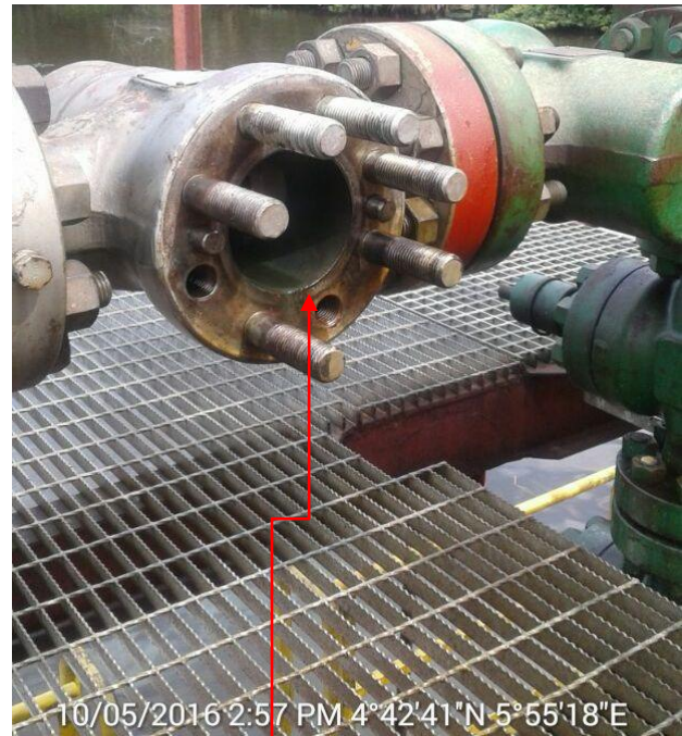
Fig B: Tampered Point, CCU missing.
