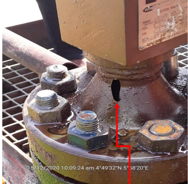
Fig B: Rupture on the Well 7 choke box
