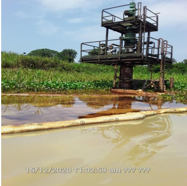
Fig A: Incident Facility (Ogboinbiri Well 7 TBG)
